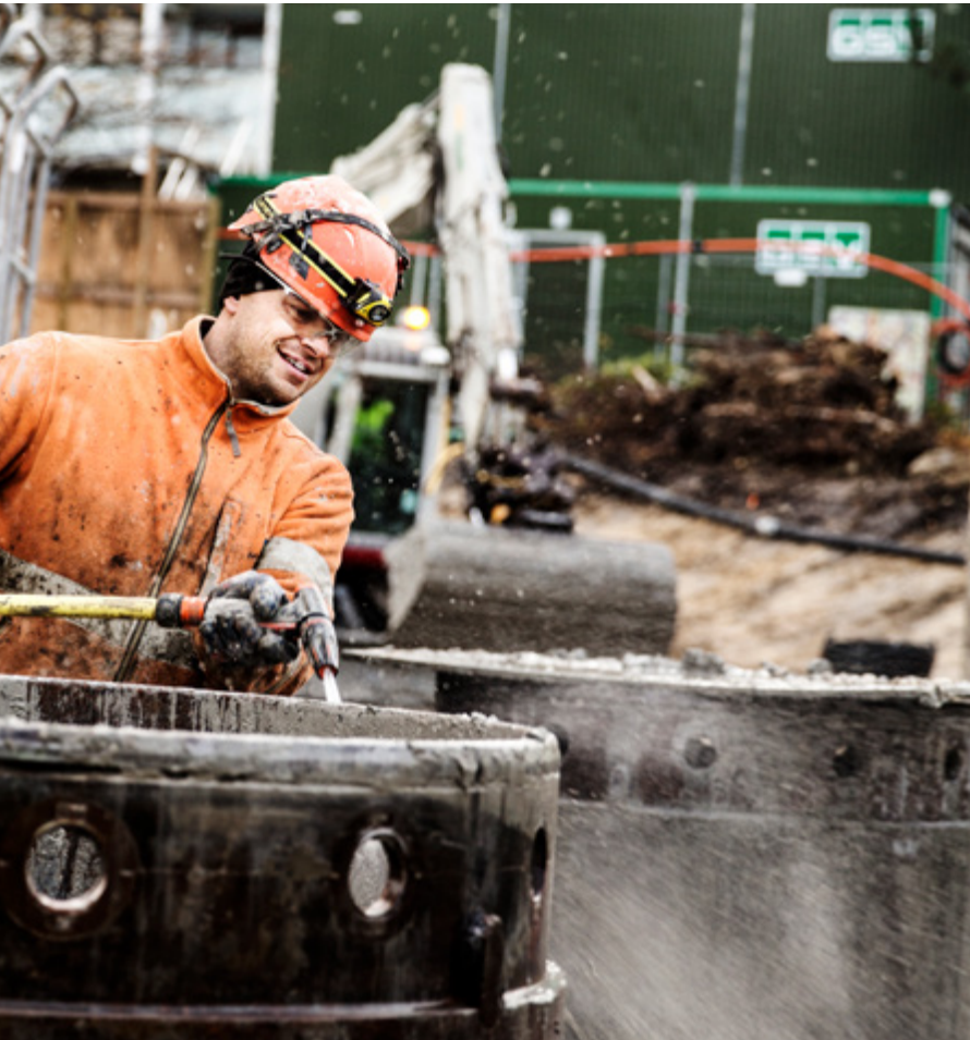
At Lyngby Station, the construction of two new tunnels under the tracks was a major task in 2019. Photo: Ditte Valente
